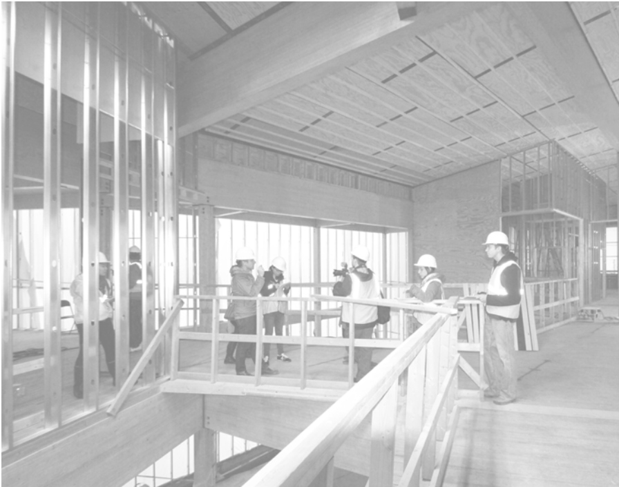
Voices from the Field Living Building Site Visit to R.W. Kern Center with Bruner/Cott Architects
